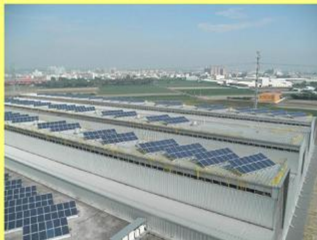
Solar Panels on Kaohsiung MRT Engine Room
